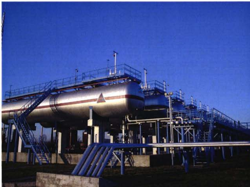
Picture 2.3 LPG terminal Batumi
