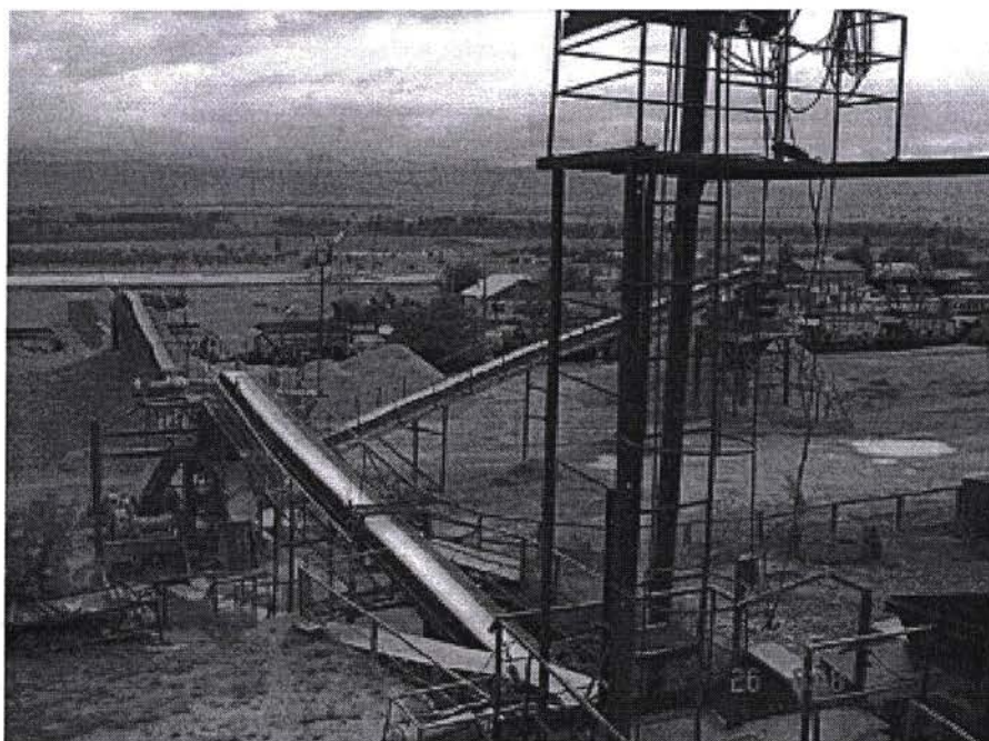
Figure 2.7 - 2 – Existing crushing plant
