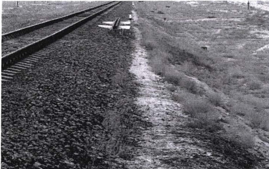
FIG. 3 Ballast view. It is possible to see that the shoulders of ballast on the sleeper side has to be slightly corrected.
