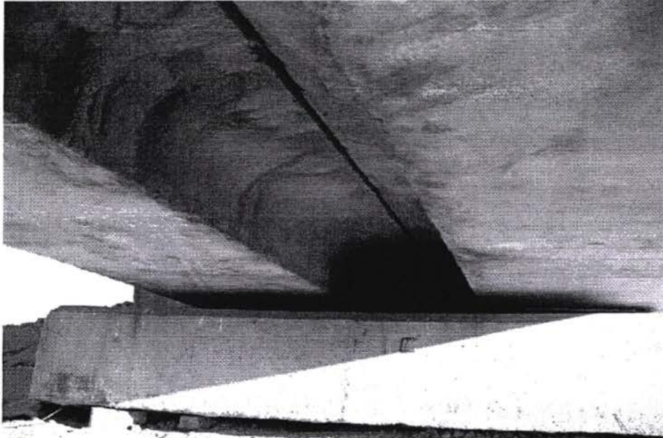
FIG. 28 Structures. 2 by 6m span hydraulic bridge. Under deck detail. The two beams are visible.
