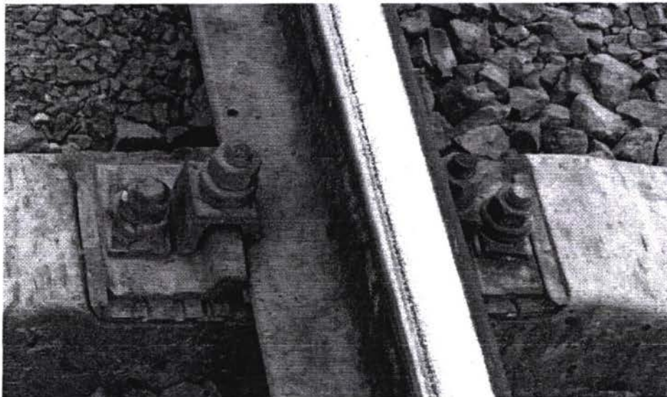
FIG. 4 Permanent Way detail in a renewed section (R65 and concrete sleeper): indirect standard fastening device and rail. As it is shown, the standard rail cross section is consumed in the inner side.
