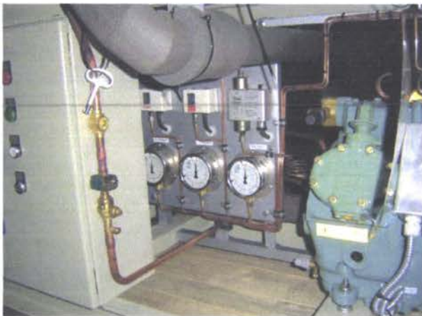
Air conditioning unit, instrument panel
