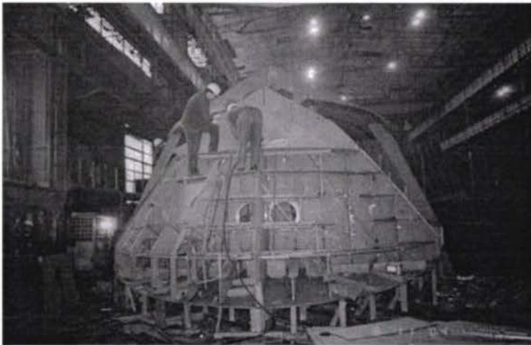
View of complete bow frame setting with foreship section still upside down
