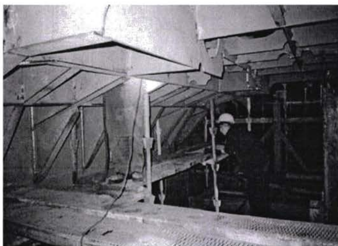
Framing stern section seen from inside engine room space with aft ship section still upside down
