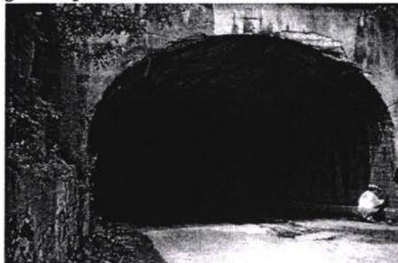
Lining of the near – portal section at the beginning of the tunnel.
