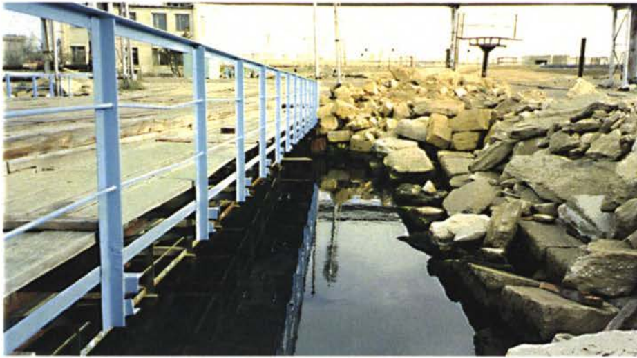
12- Poor slope protection.
