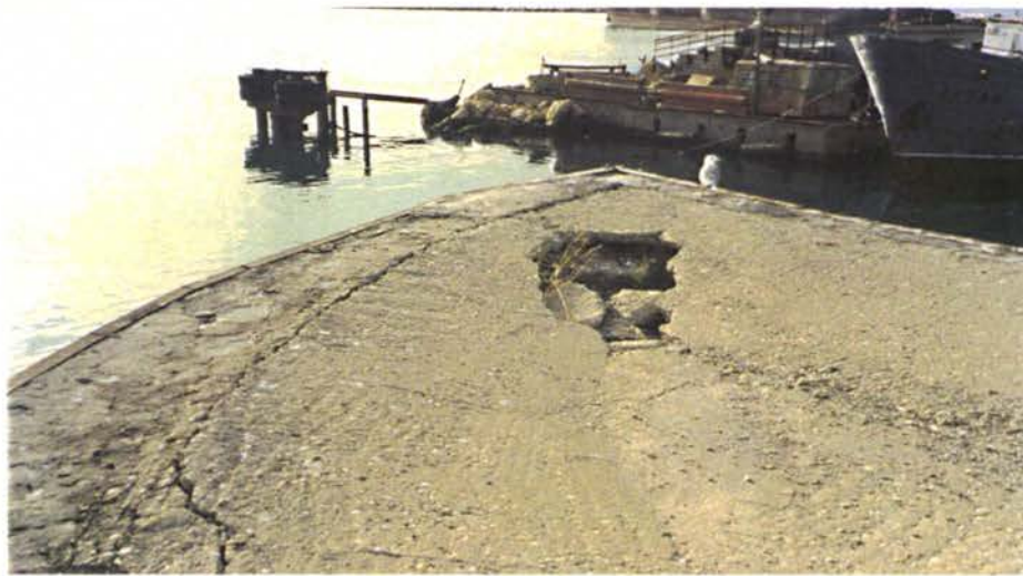
13- Cracked concrete pavement at the head of finger pier.
