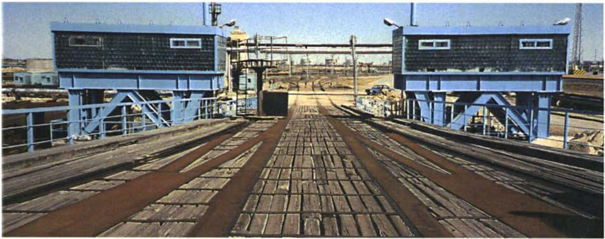
1- Ramp deck and inner lifting towers (notice aerial oil and water pipes).
