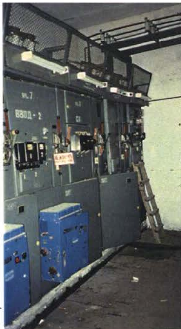
22- Electrical panels inside transformer substation TP 803.
