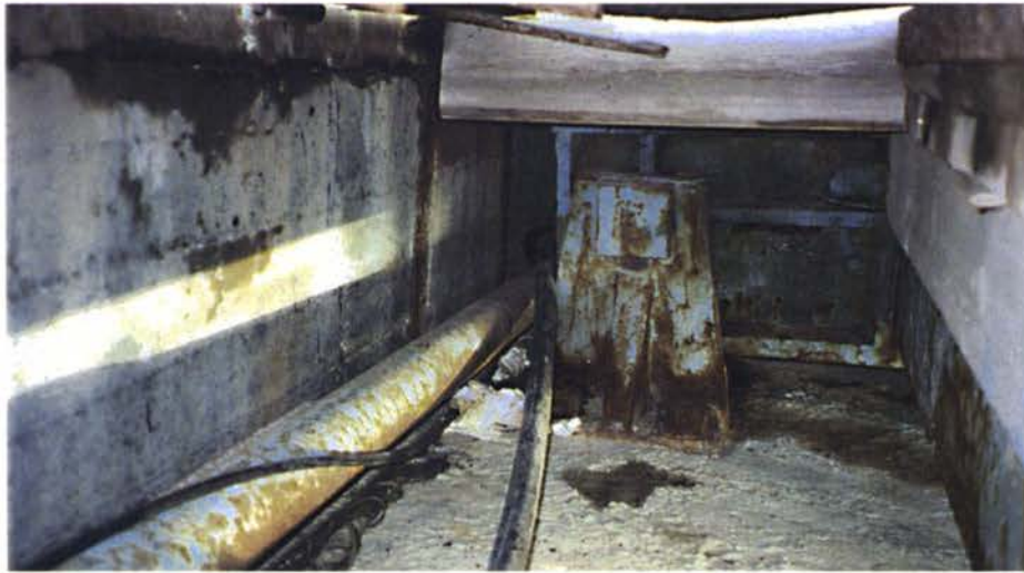
16- Corroded pivot bearing on shore base (starboard).
