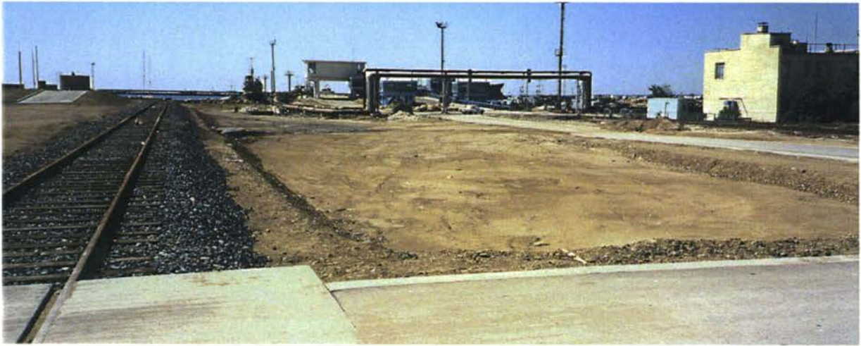
4- Ferry parking area and access road to the ferry ramp (the rail-track was rebuilt under phase 1 programme).
