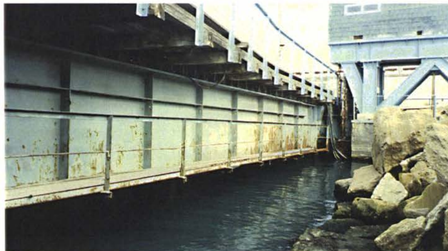
17- Corroded ramp guider.
