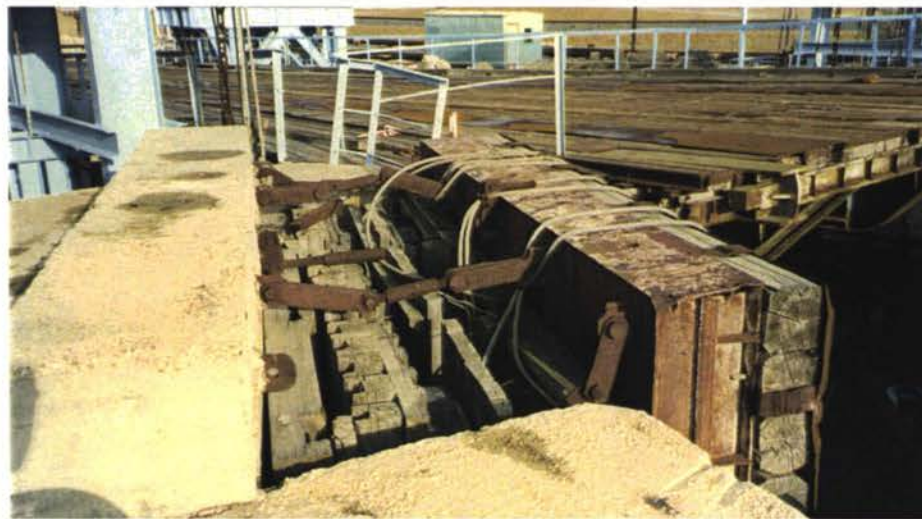
14- Broken arms on starboard stop fender.
