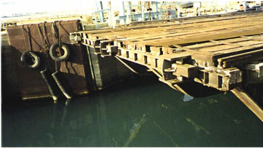
15- Poor fendering on starboard stop fender.
