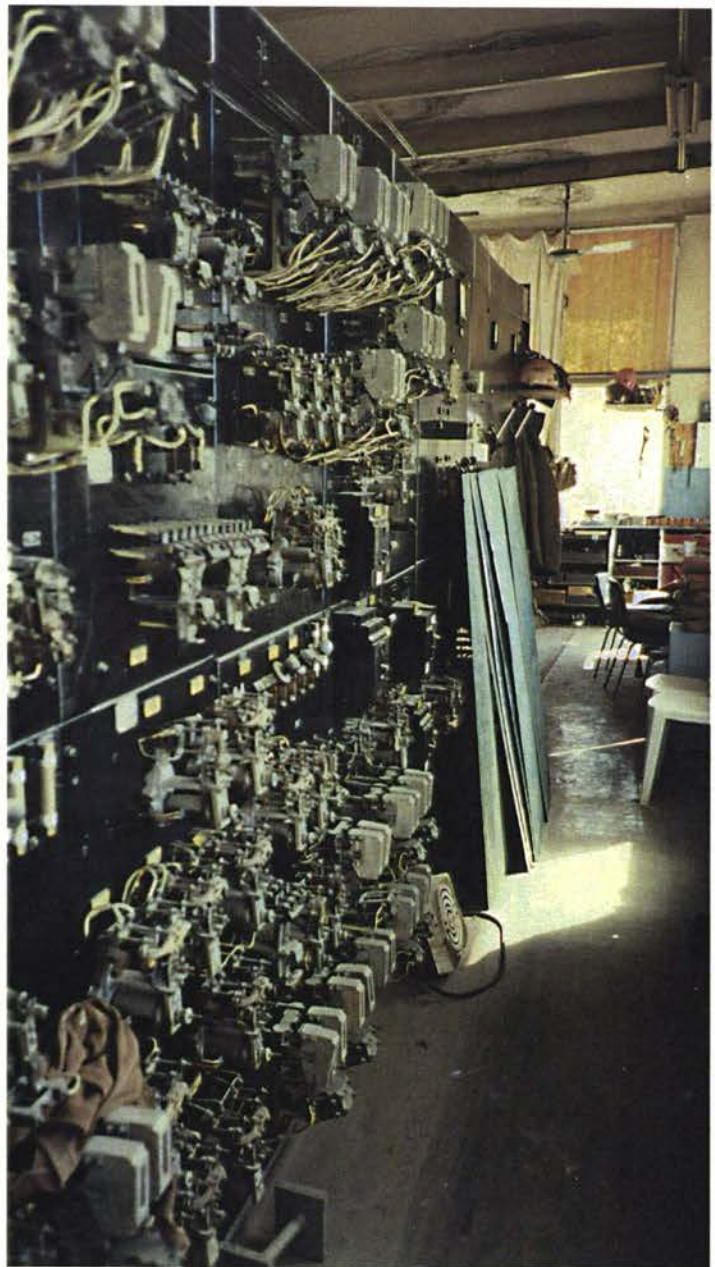
19- Control boards in central control tower.
