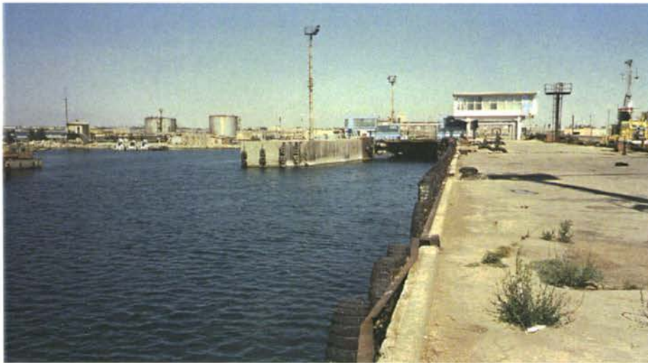
10- Damaged pavement on central pier.
