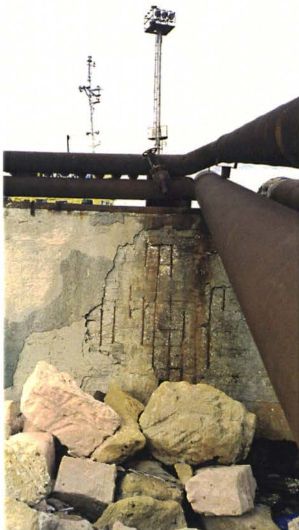
8- Eastern side of central pier (old oil loading pipes and damaged concrete).
