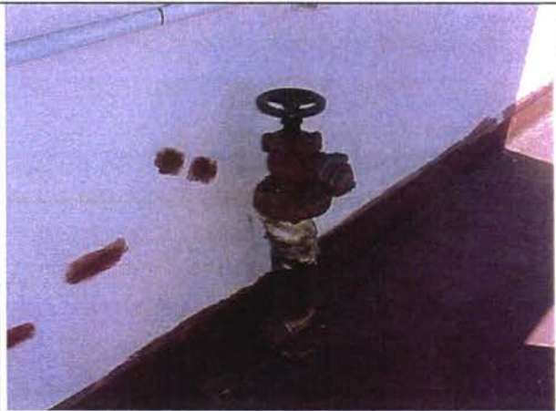
Hydrant, handle cannot be turned
