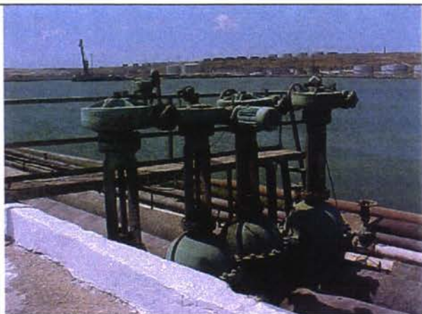
Valve system for pipe lines
