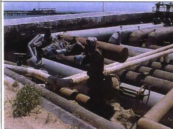
Pipeline and fire fighting system on pier 1, no water supply, seals partly broken or off, valves can be turned
