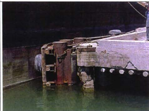
Broken concrete pile of pier 1 and fender system
