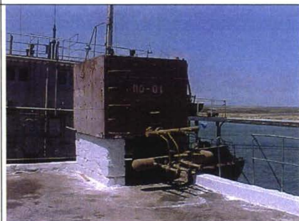
Tank system for fire fighting foam on pier 1
