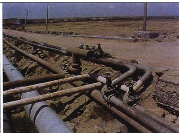
Pipeline from shore side to pier 1, 2 and 5 for fire fighting
