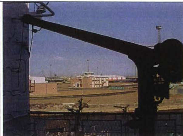
Portside crane behind lifeboat, out of order
