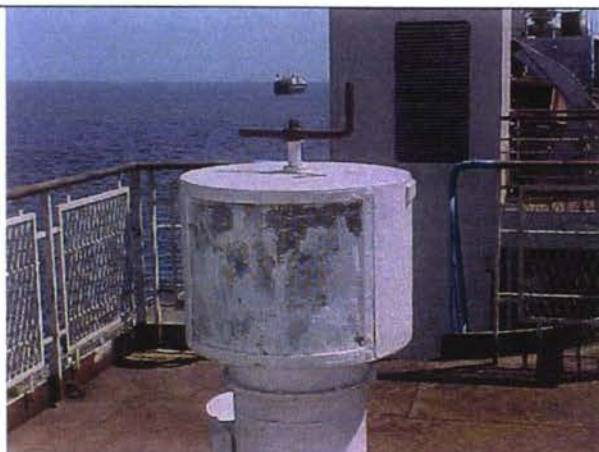
Ventilation, spindle can be turned, sieve partly painted
