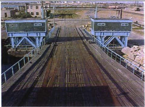
RoRo ramp in Aktau, the rails are covered with timber, railway operation not possible
