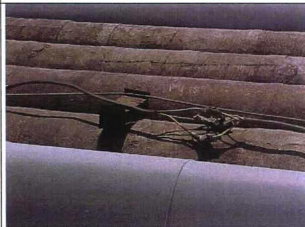
Pipeline from pier 1, 2 and 5 to shore side with electrical cable
