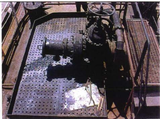
Manifold of tanker " General Heydarov", 4987t, arm disconnected
