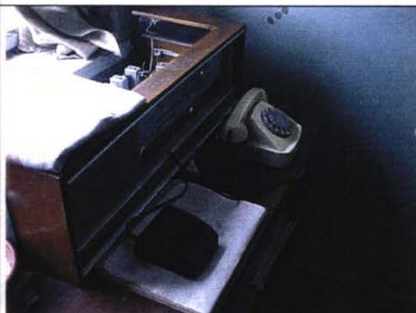
Additional equipment of Port Control Centre Dubendi, battery charger, telephone and radio for warnings
