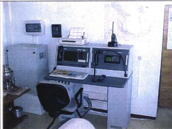
Wireless station from Raython with telex, VHF, MW, GMDSS and hand held radio with restricted channels
