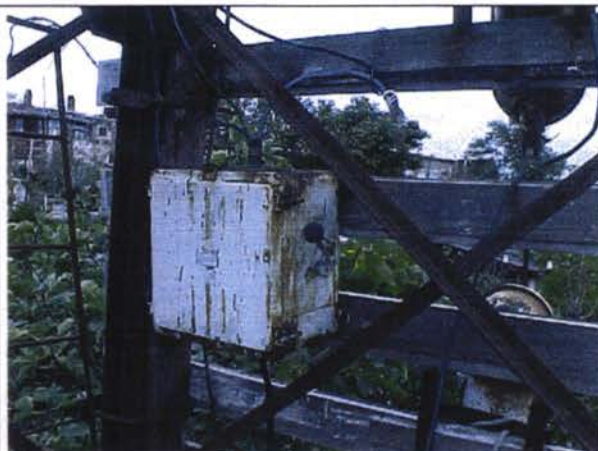
Tower 1: Distributing box
