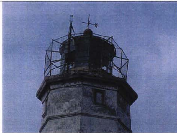
Lighthouse Narjin: View to the upper part of the light house with broken window pane and damaged mantelpiece
