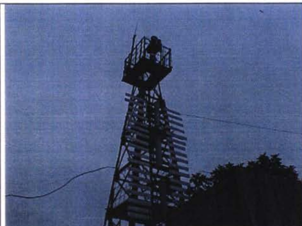
Baku Leading Lights Tower 1: View from the south west side with look to the electrician supply cable
