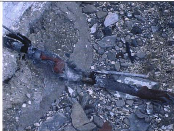
Unconventional out door cable connection (220 Volt) between generator building and light house
