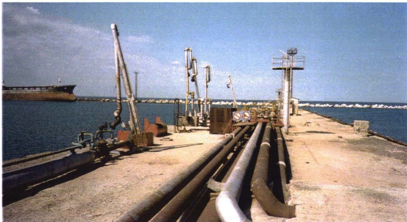
7. On pier top: pipelines, loading arms and water cannon (June 2001)
