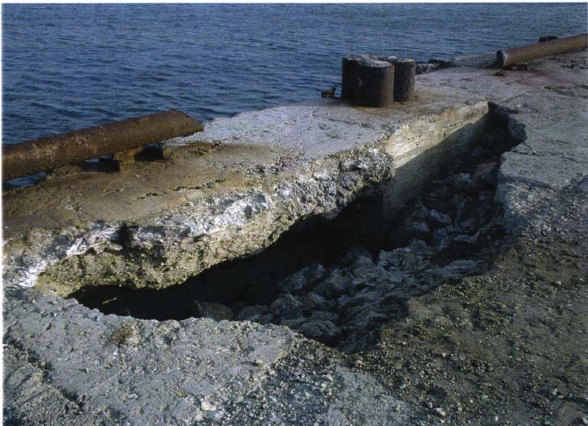
6. Cavity behind berth n°5's bulkhead (year 2000, prior to temporary repair works)
