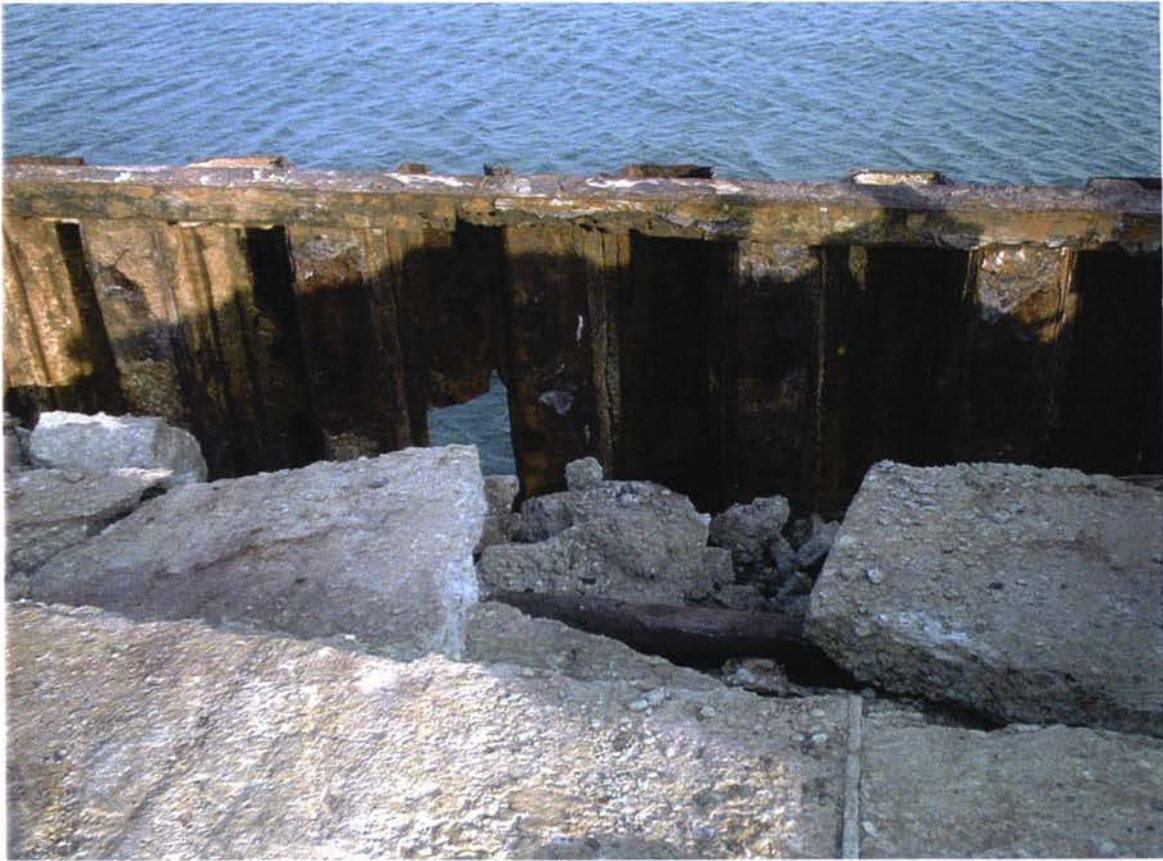
5. Perforated sheet-pile at berth n°5 (year 2000, prior to temporary repair works)
