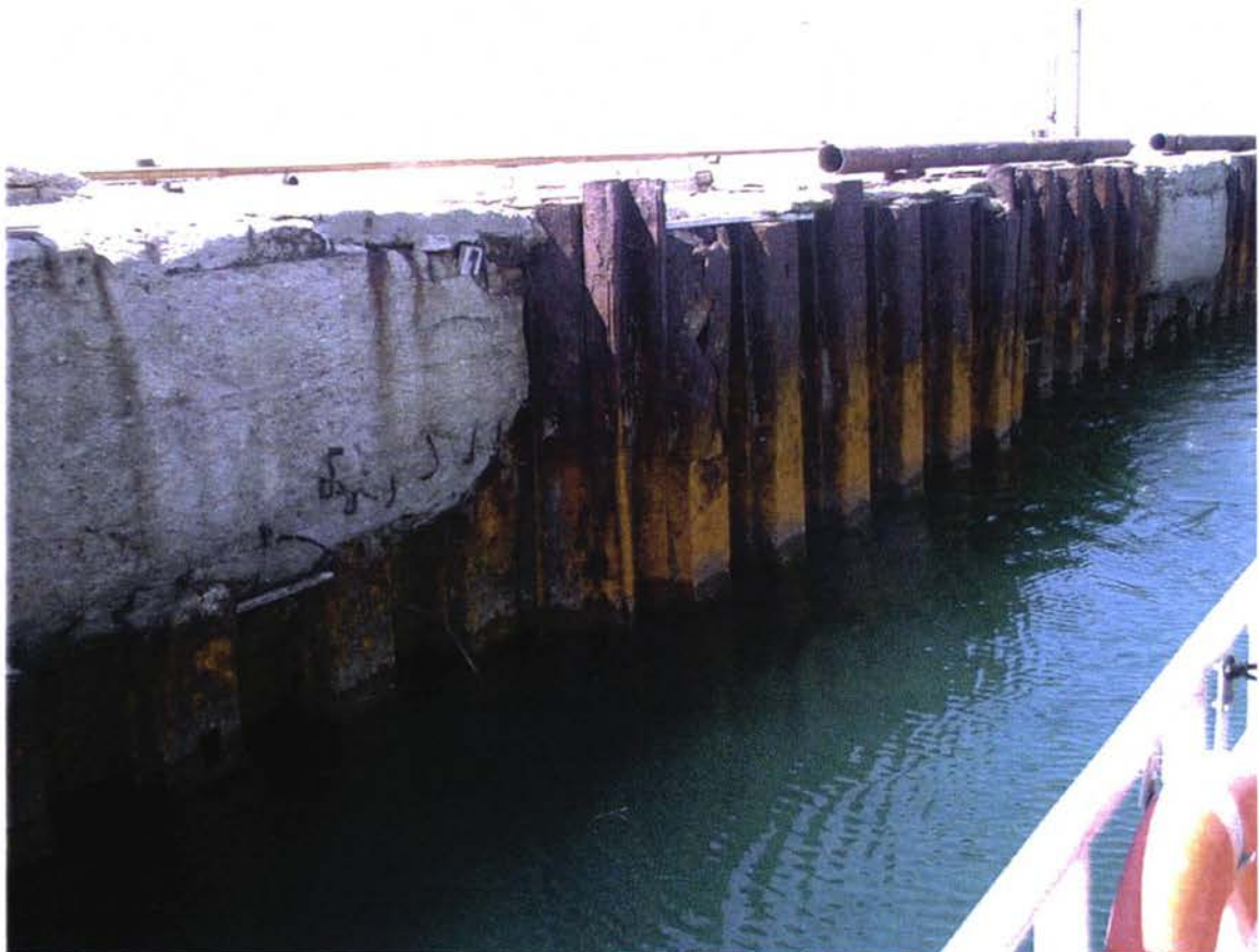
4. Corroded sheet-piles and worn out capping beam - berth n°5, June 2001
