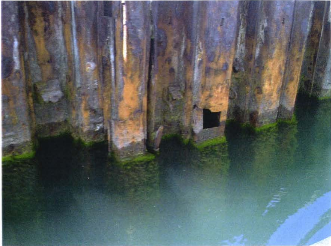
3. Corroded sheet-piles at berth n°5 (June 2001)
