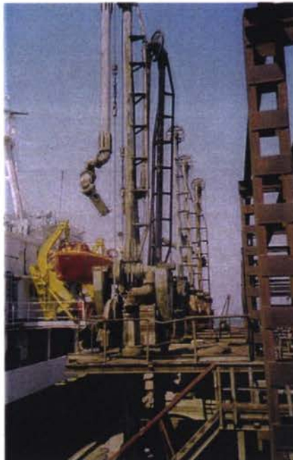
17. Pier n°3. Unused arms for refined oil
