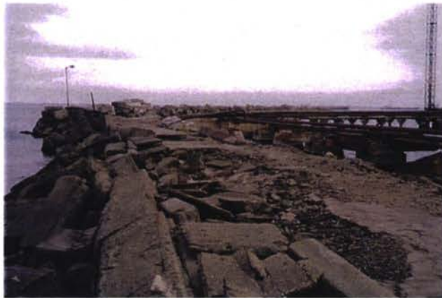
5. The most damaged part of the breakwater, between pier n°2 and pier n°5
