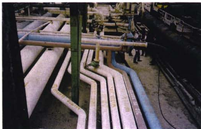
9. Pipe nets on pier n°1
