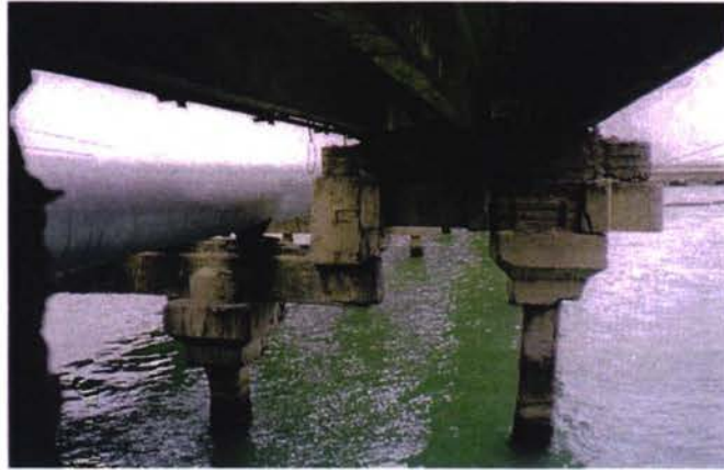
10. Underneath pier n°1 (damaged reinforced concrete)
