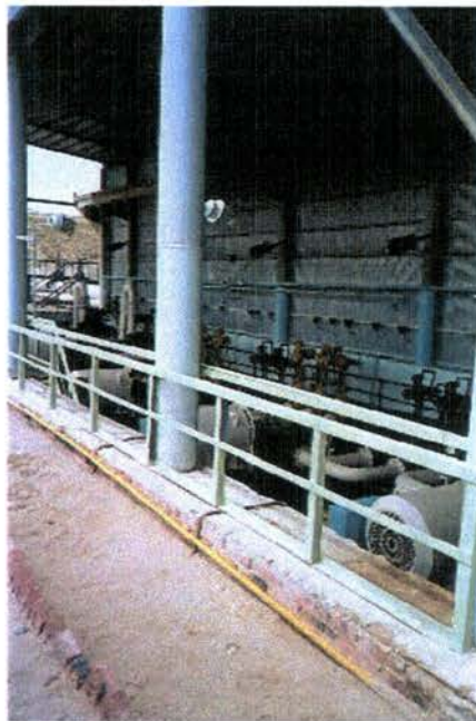
22. Caspian TransCo pump station
