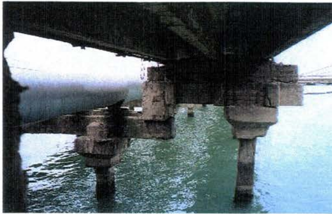
10. Underneath pier n°1 (damaged reinforced concrete)
