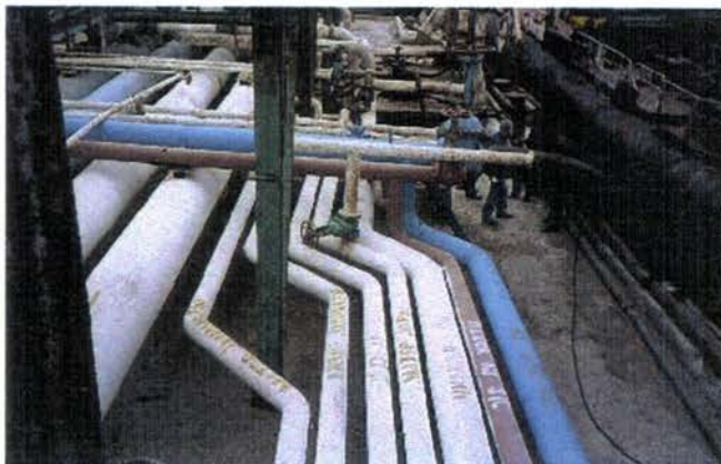
9. Pipe nets on pier n°1
