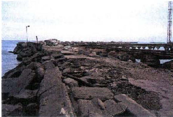
5. The most damaged part of the breakwater, between pier n°2 and pier n°5
