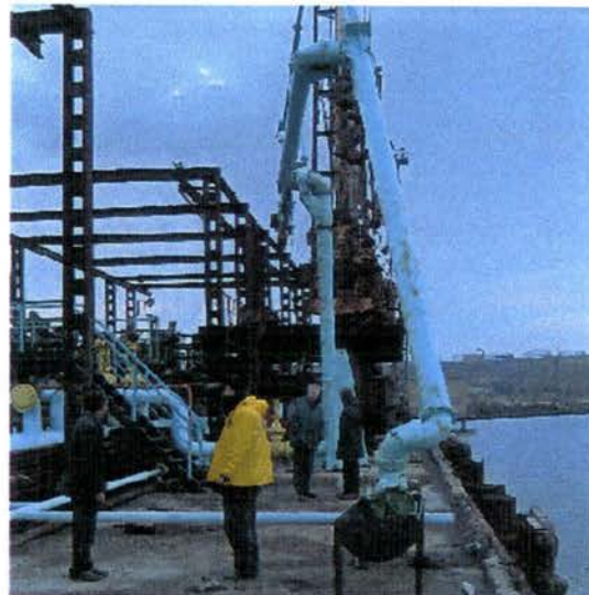
18. Pier n°3. Brand new arms for unloading crude oil
