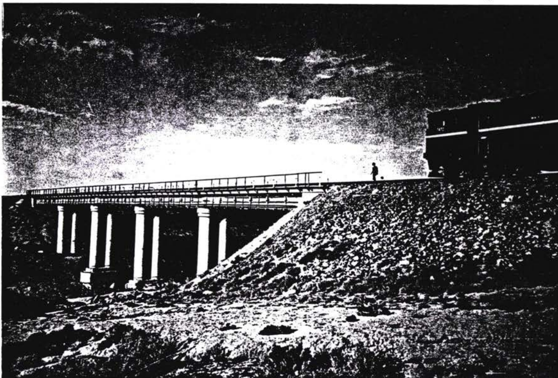
Bridge at km 339,5 This bridge was build up 1993 after the old one was distructed during a rainfall
