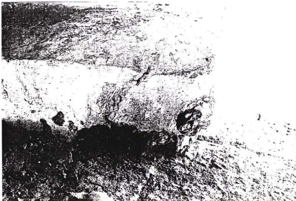
F7-30 Span 26 Bearing A1 - crack
